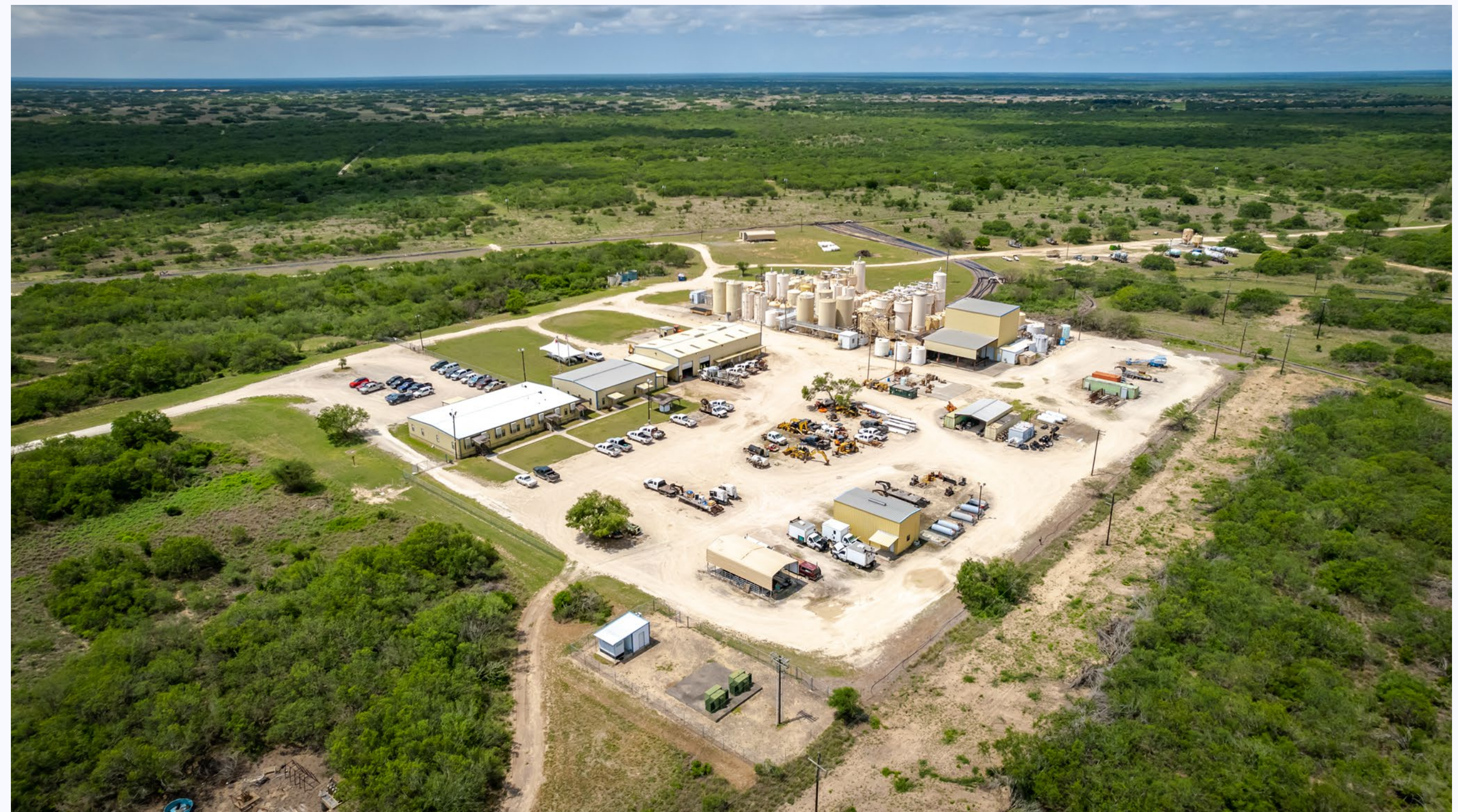
Alta Mesa Central Processing Plant
