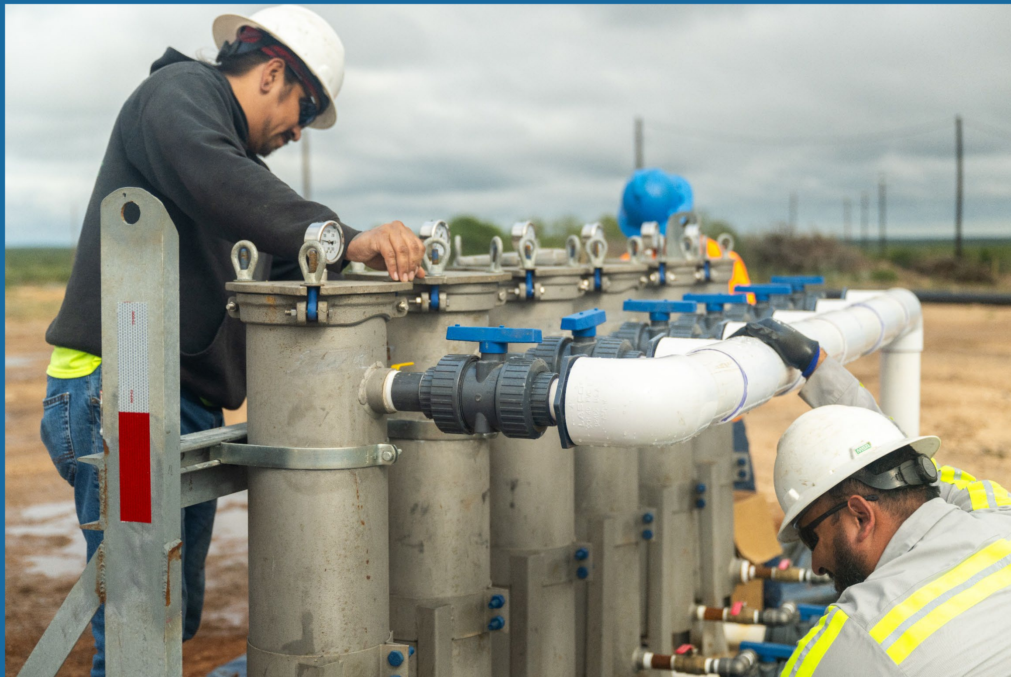
Rosita ISR Uranium Central Processing Plant
