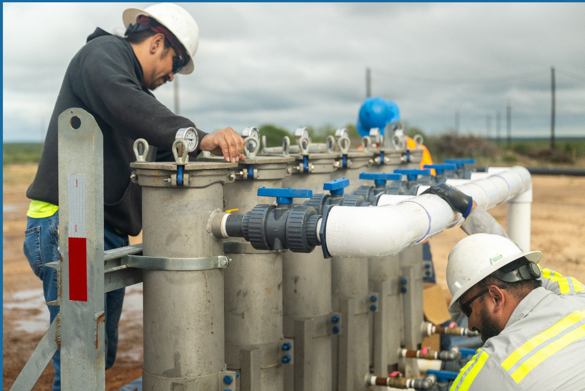
Rosita ISR Uranium Central Processing Plant
