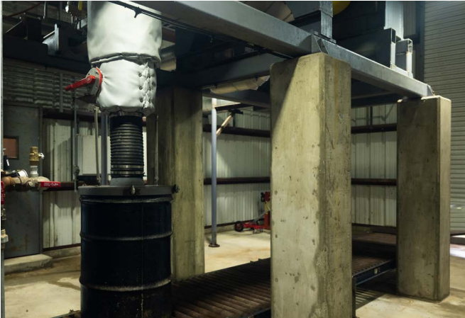
Dryer at the Rosita CPP ▲
